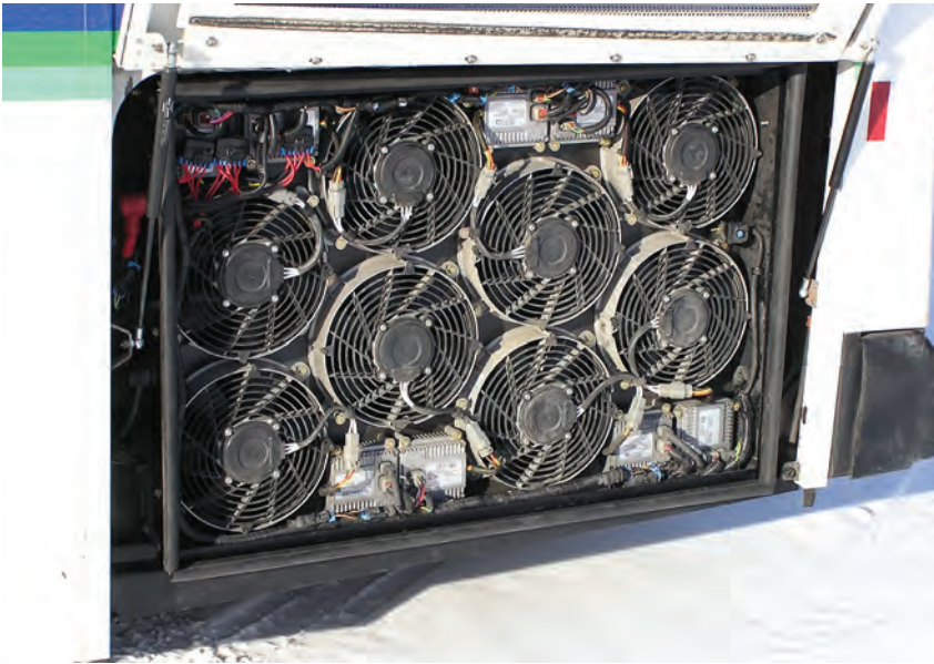
EMP's retrofit cooling system is also now in pilot testing with several other transit fleets. Shown here is a bank of Diesel Grade fans being adapted to a bus operated by the Capital Area Transit Authority of Lansing, Mich.
